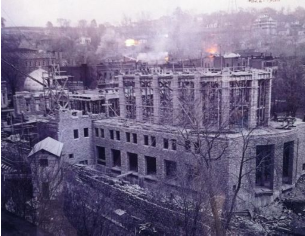
Fig. 1 Photograph of the Hall of Waters under construction, Nov. 6 1936. Source: Hall of Waters history exhibit in the Hall of Springs.
